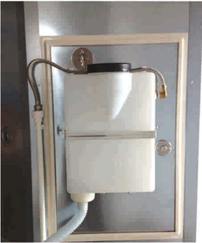
Reservoir system is outside of wet unit walls.
